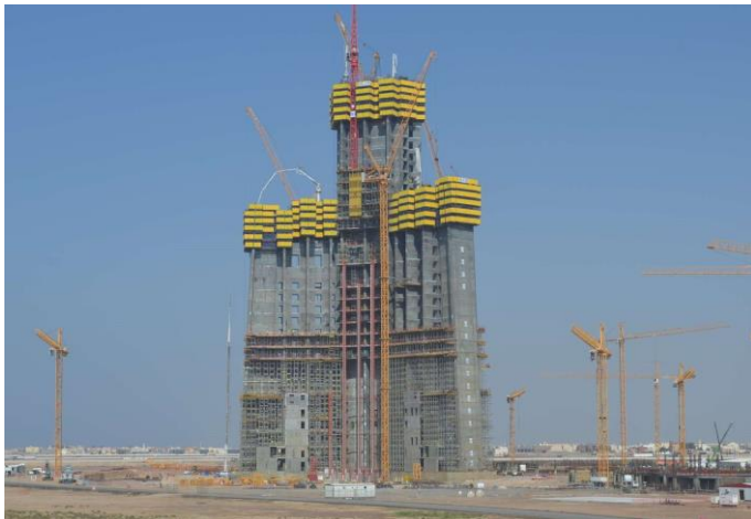
Our reference in Jeddah, Western Region (Kingdom of Saudi Arabia): Kingdom Tower Picture Source: Google Maps.
